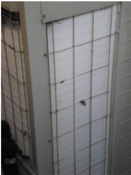
Left: Frost build-up on air source
