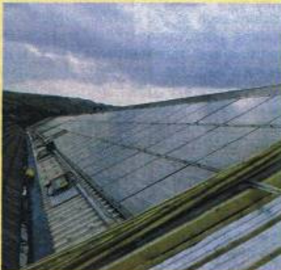
Solar photovoltaic panels, together with a biomass-fuelled CHP system, provide renewable energy on-site
